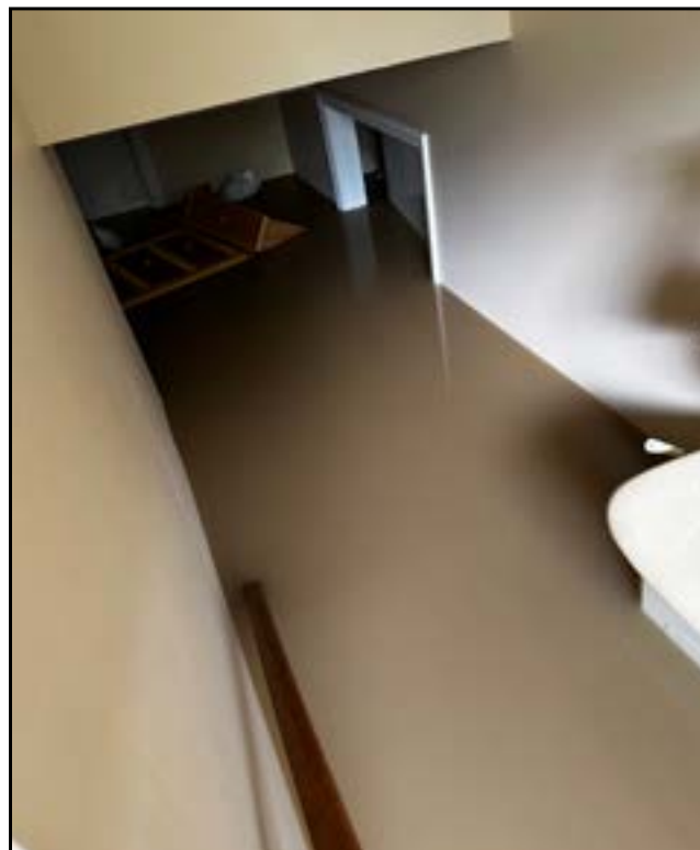
Murky brown flood waters fill the basement of Maddy's home.
